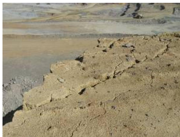
Figure 9. Ice formations and accumulations of water on safety berm on the southern pit wall in the ramp area (April 2012) and cutter breaks on the western pit wall on the +200m level
