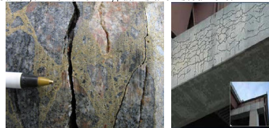
Figure 1- some samples of cracking because of stones Alkali reaction.
