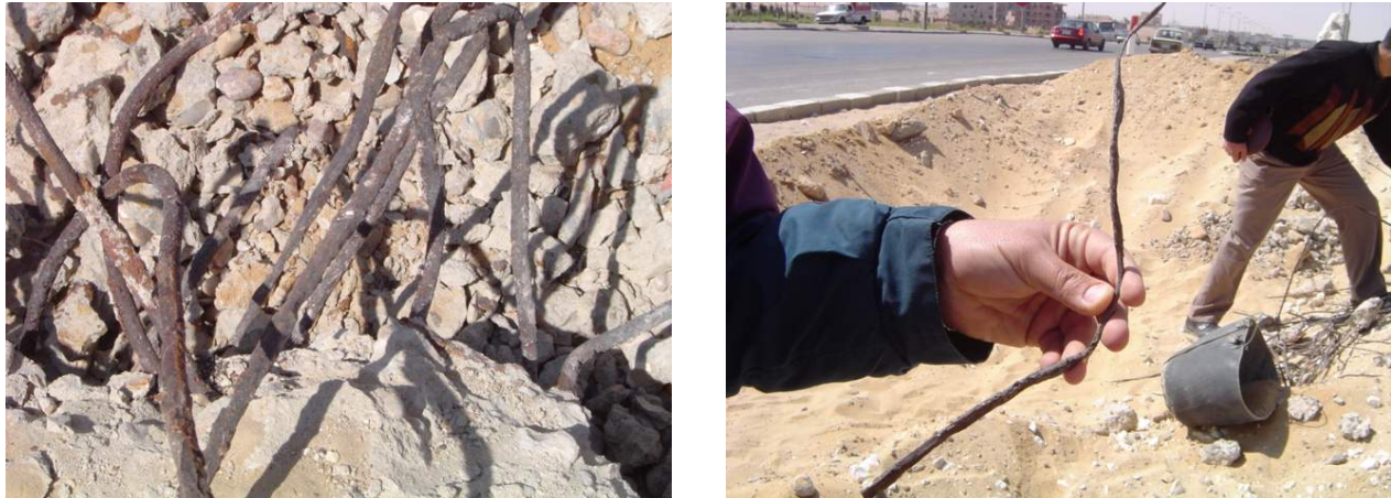
Figure 7: Example of corroded rebar
