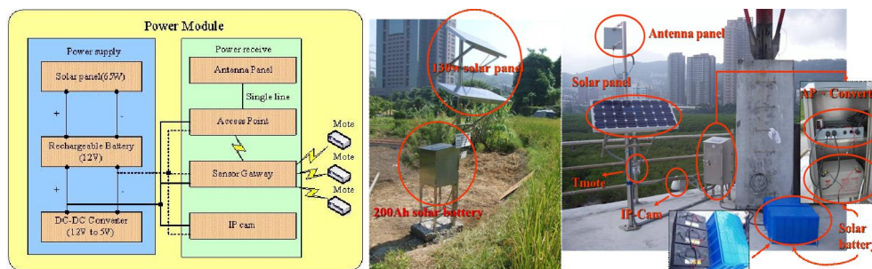
Figure 8. Power module and Gateway node in SS1 and SS2
