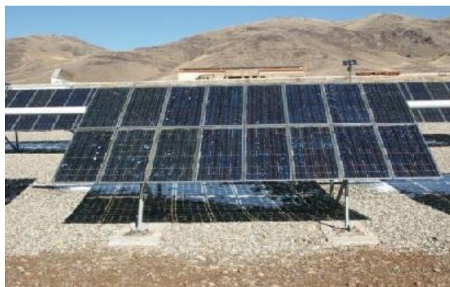
Figure 1, Photolytic 10 kw capacity Power Plant
