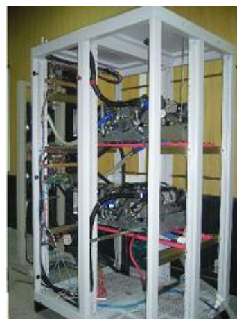
Figure 6 Implements of 25 KW Fuel cell project
