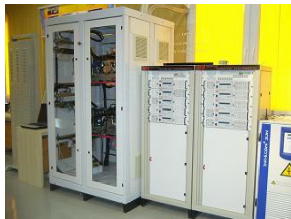
Figure 5 Implements of 25 KW Fuel cell project
