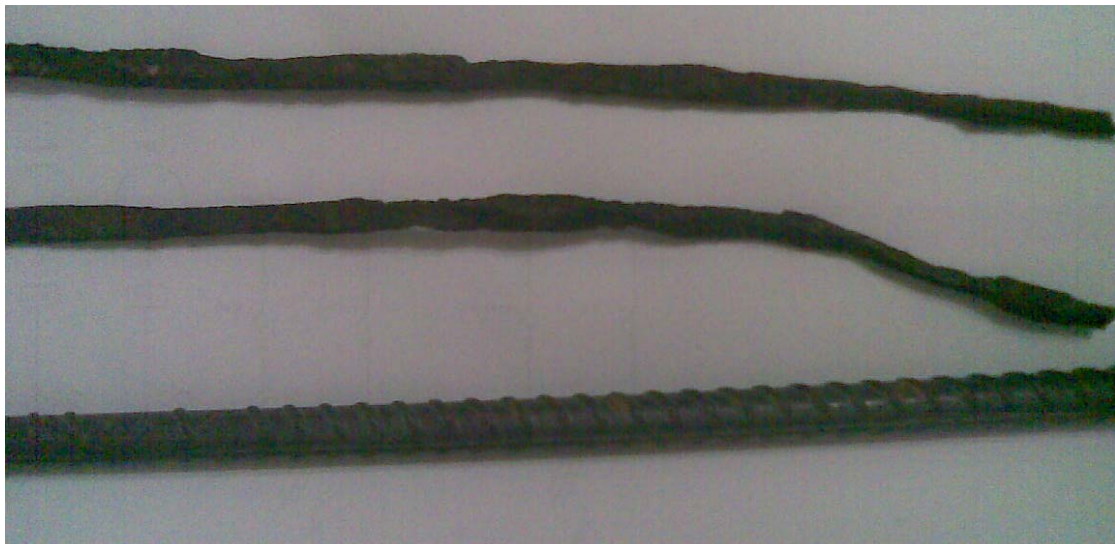
Figure 8: Comparison between rebars before and after metal loss due to stray current electrolysis
