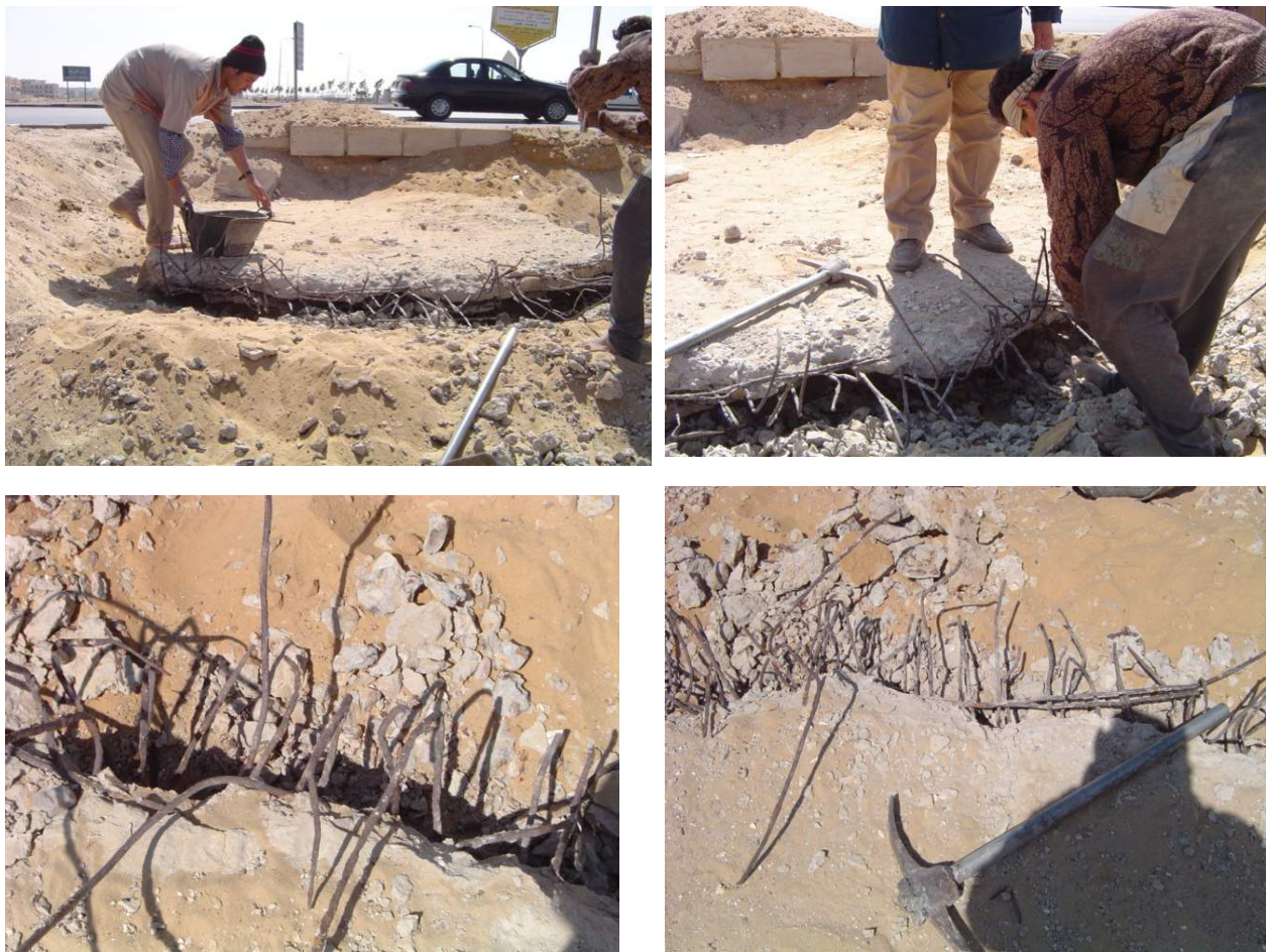
Figure 6: corroded rebars were subjected to the cathodic zone of SUMED pipeline
